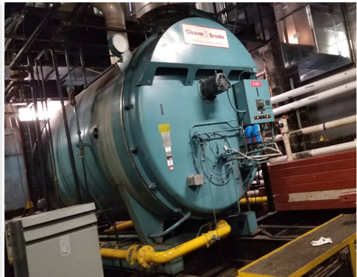
Figure 3 Steam boilers currently in use
